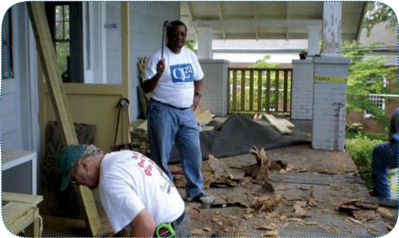
Volunteers Robert Fletcher (above) and Pam Cook (lower right) help to refurbish a porch for Homes of Hope, a Compassion Coalition designated assistance program.
